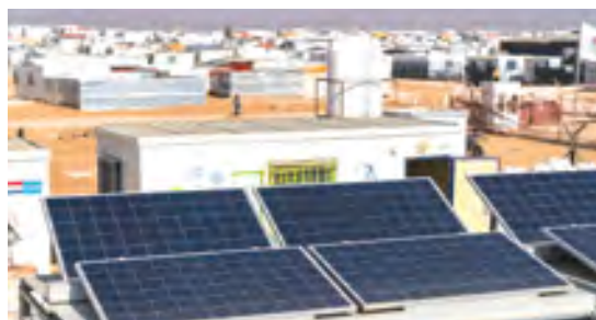
Solar panels, Za'atari Camp, Jordan
