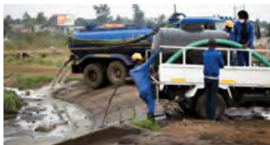
Sewage discard from a truck tank into the Infulene Waste Water Treatment Plant, Maputo, Mozambique
