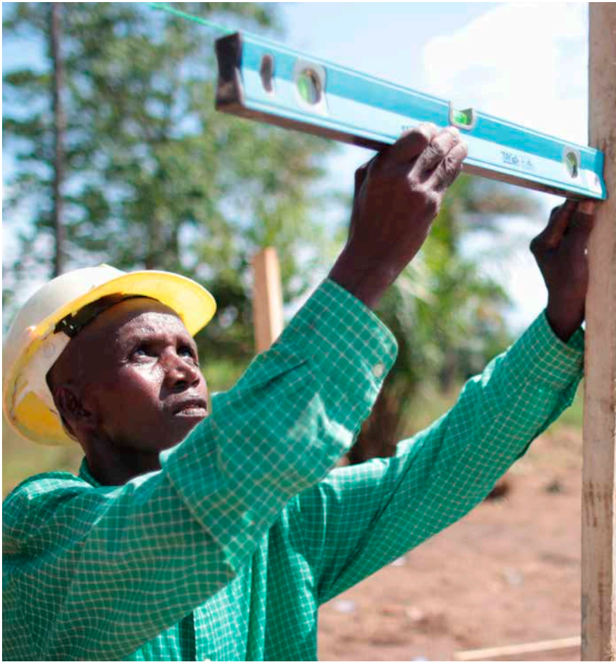
▲ Sierra Leone: A builder constructing an eight bed Community Care Centre in Pate Bana, Bombali district
